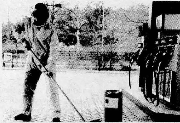
Fig. 1 - Sealing Pavers on petrol station forecourt
