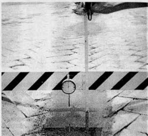
Rutting of some 100 mm a long the transtainer track - where CBP placed Directly on top of the old Asphaltic pavement
