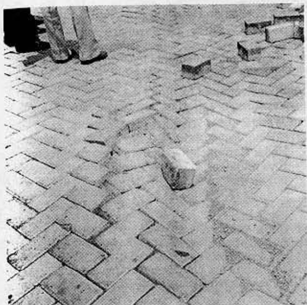
Surface damage of the CBP due to excessive dropping of loaded containers from some high by top loader.
