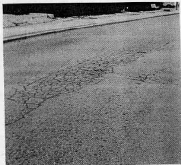
Fig. 2: A picture of alligator cracks and rutting in the asphaltic pavement.
