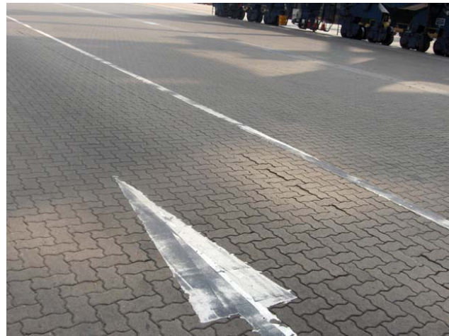
Figure 10. Defective Area (YICT)
