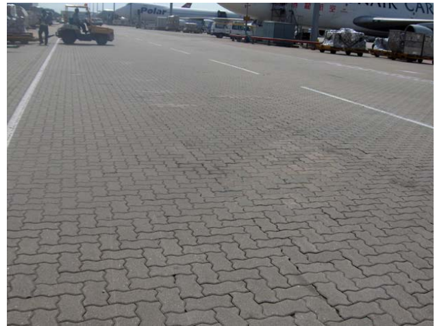
Figure 6. Defective Areas (HKIA)
