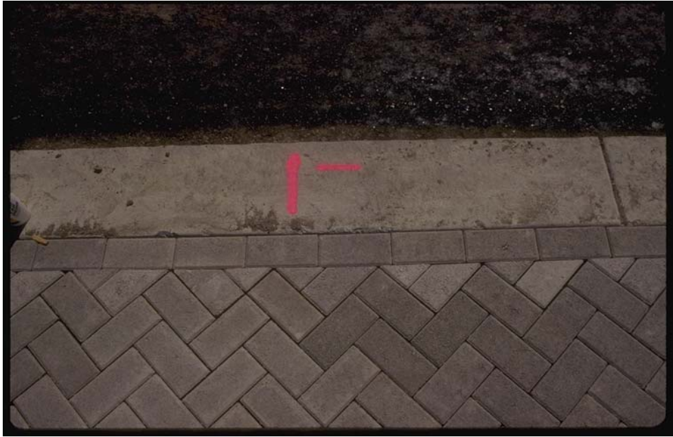
Figure 8: A row of full pavers against the restraint gives a better visual appearance and increases the performance of the pavement Source: Interlocking Concrete Pavement
