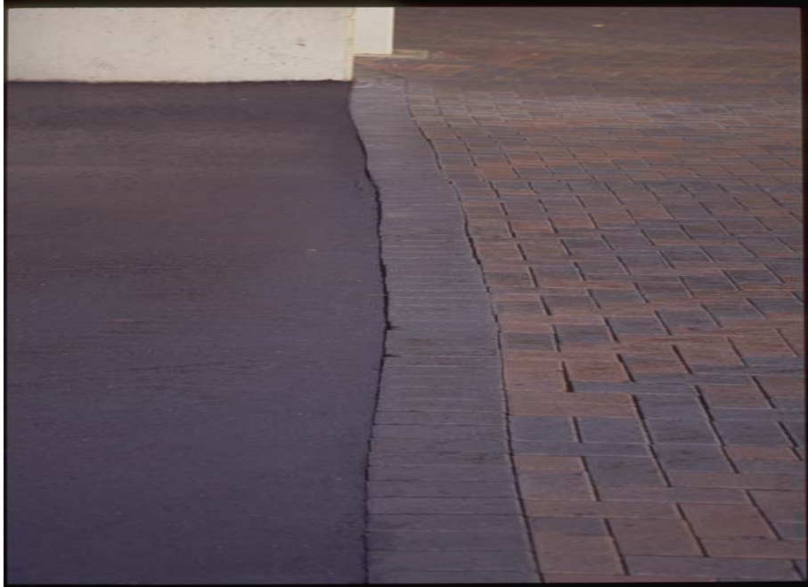
Figure 15: The stress on asphalt beside paver crosswalks can cause it to deform or move away resulting in reduced interlock and potential deformation of the pavement. The designer should consider reinforcing the asphalt edge with concrete and should ensure an adequate thickness for the asphalt restraint
