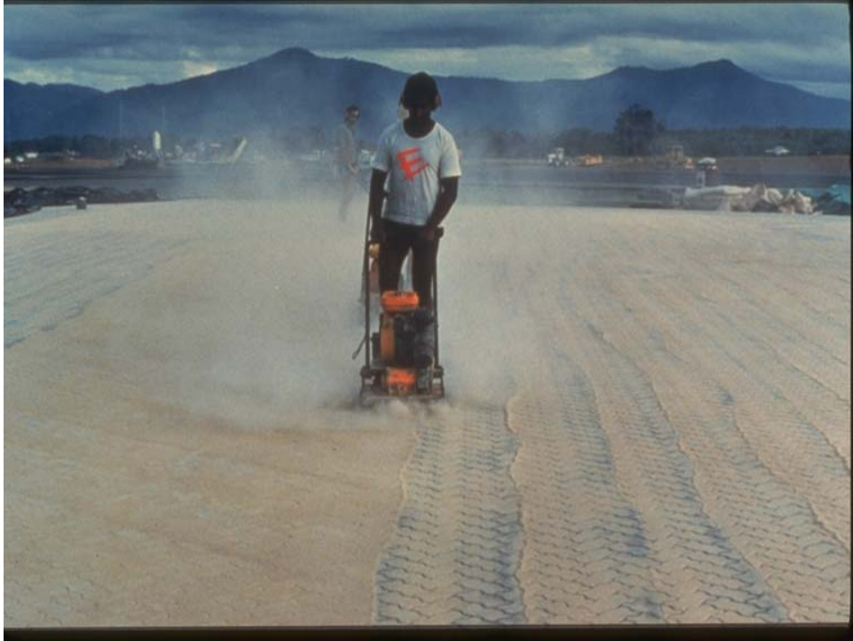
Figure 6: Joint sand is applied and the pavers go through a final compaction Source: Interlocking Concrete Pavement Institute
