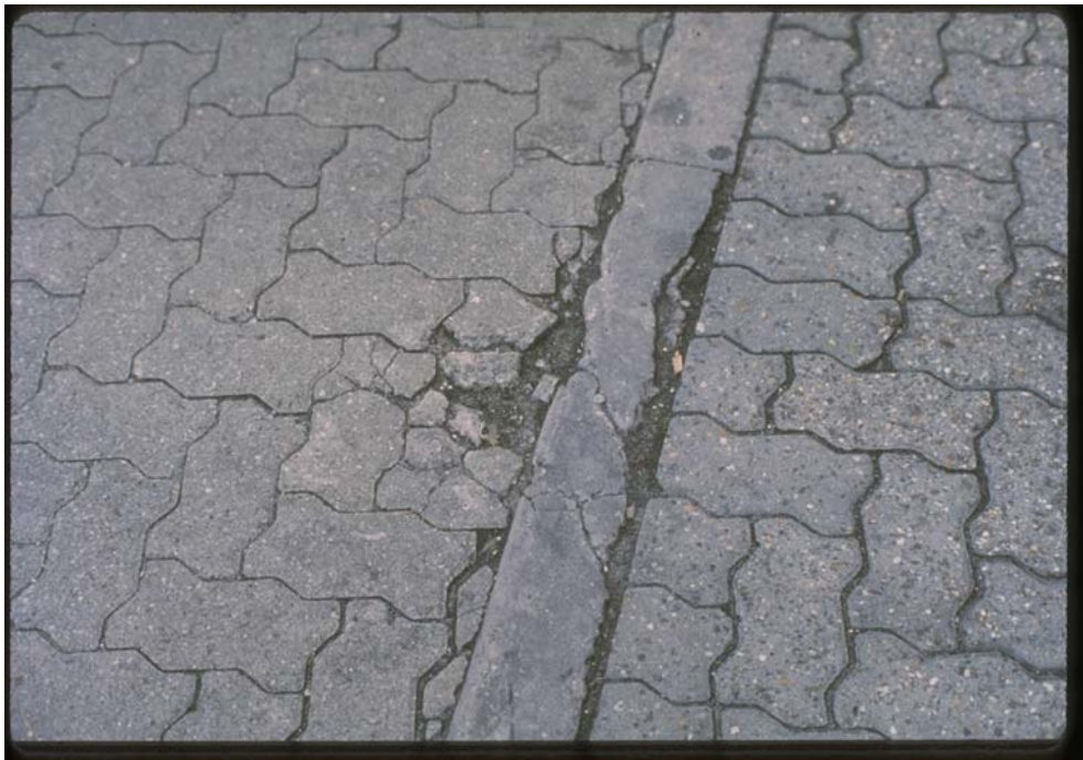
Figure 9: In this vehicular application, the pavers on the left were cut and placed at less than 1/3 of the original paver size, whereas the ones on the right were not. Source: Interlocking Concrete Pavement Institute
