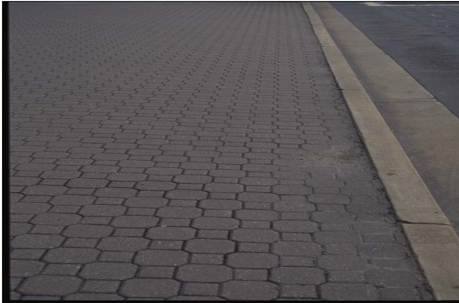
Figure 10: To eliminate settlement at the edge of curbs, backfilled materials must be adequately compacted and the density monitored with density gauges Source: Interlocking Concrete Pavement Institute
