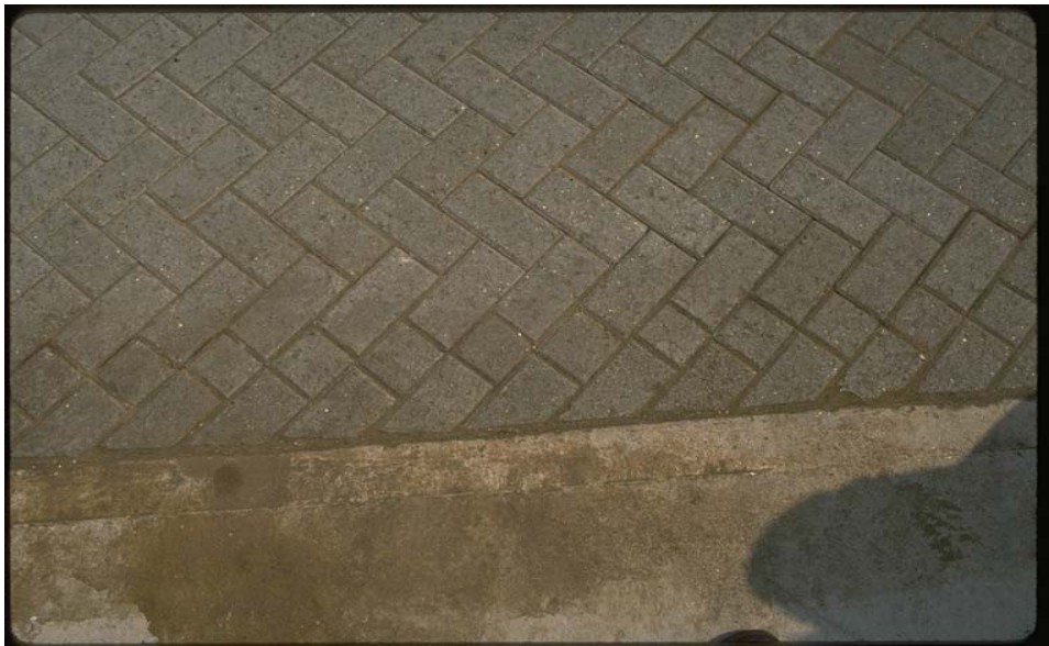
Figure 7: Pavers cut and placed directly against a restraint Source: Interlocking Concrete Pavement Institute
